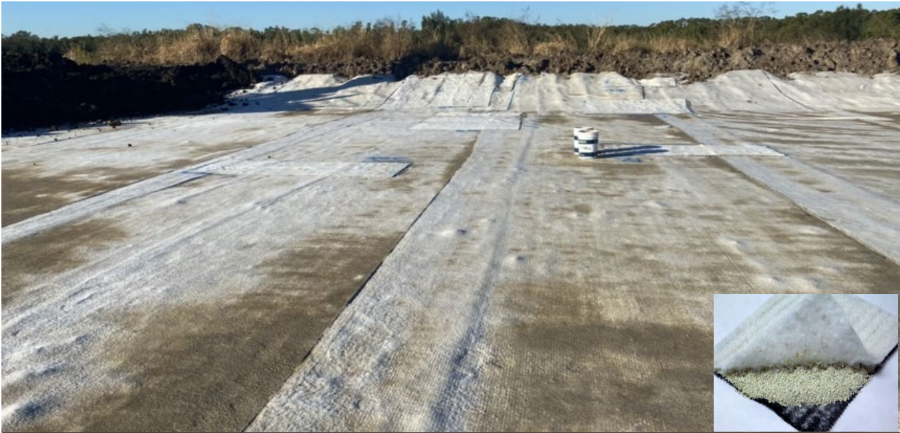
Image 7: Bio-retention basin Southern Cross Way - basin floor liner (Geosynthetic Clay Liner, see example of liner)
