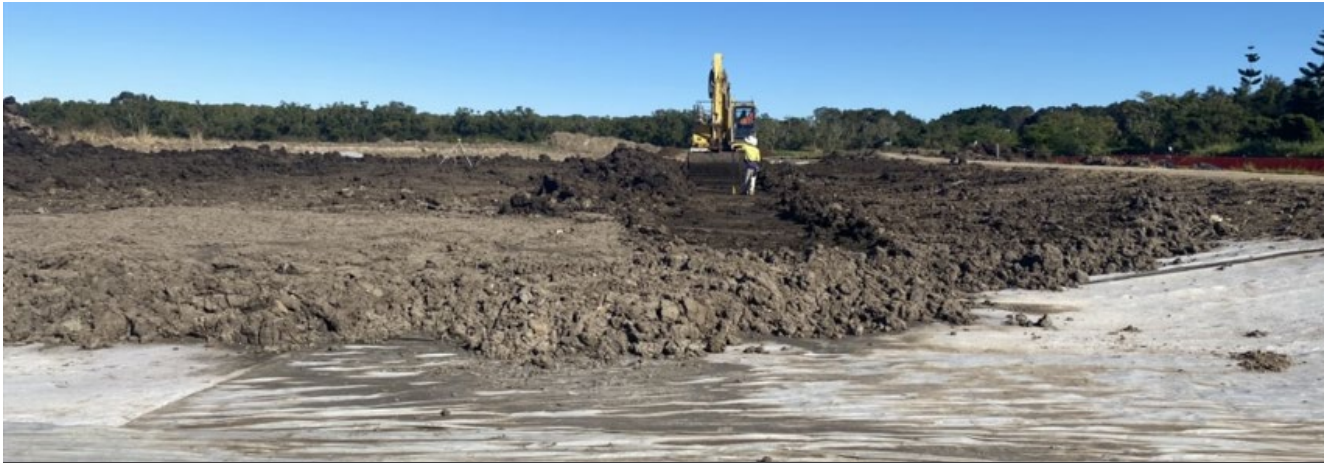
Image 9: Bio-retention basin Southern Cross Way- spreading topsoil over the basin floor liner
